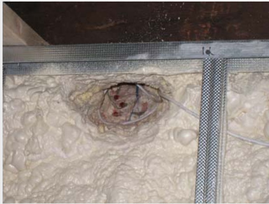
Melted wire insulation from overheating closed-cell foam
